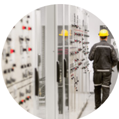
Related infrastructure for electric utilities
